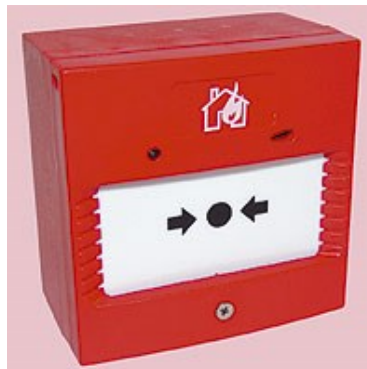
Figure 5a: A Fire Alarm Manual Call Point (Coloured red)
